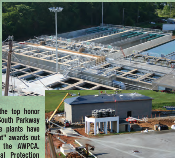
Construction at the South Parkway plant will add 12 million gallons of water per day to the systems' capacity.
